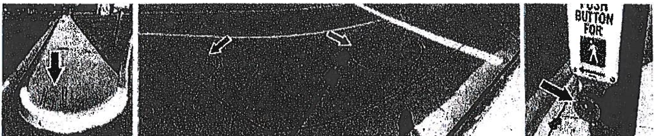
Exhibit 1 – Existing pullboxes, detector loops, and substandard pedestrian pushbutton at Adams/Pinecreek which will be relocated, modified, or replaced as part of the reconstructed southwest corner
